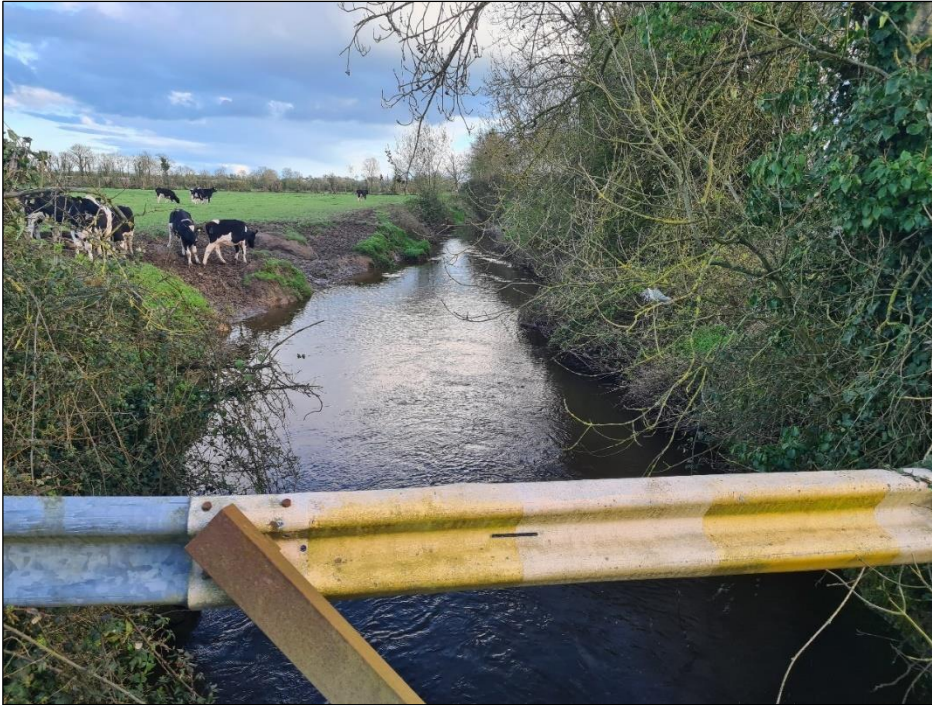
Plate 3-25 View of existing crossing at the Suir River located at the southeast of the Site leading the proposed substation location from turbine 8.
